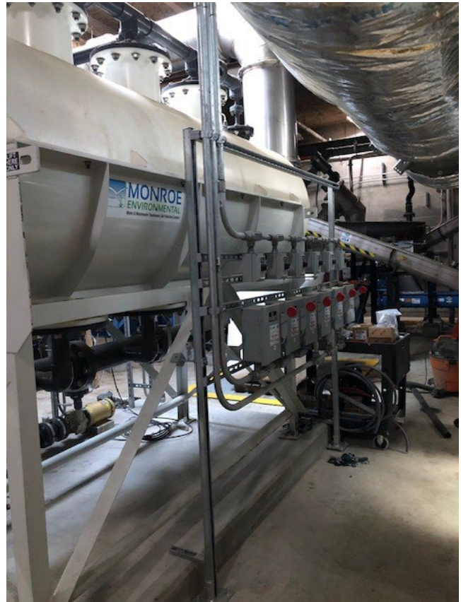
Odor Scrubber Upper level.
